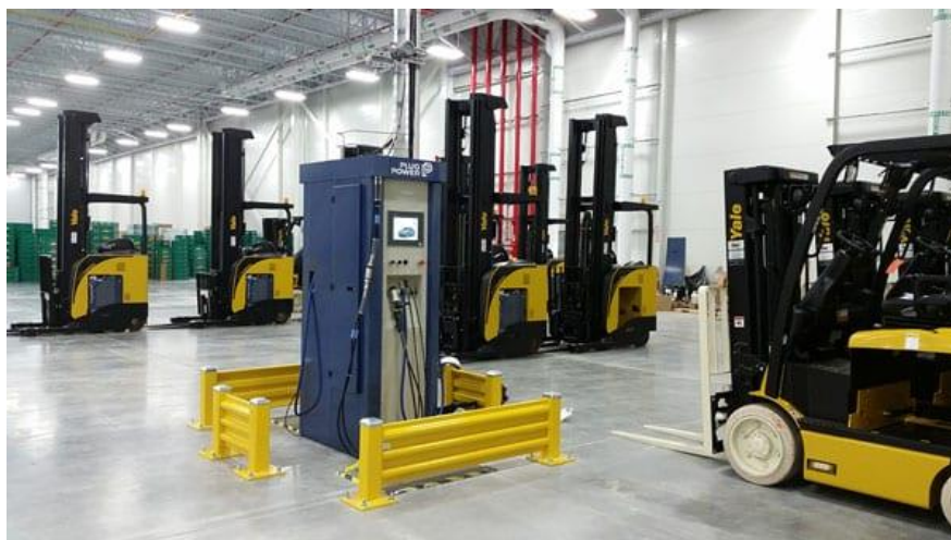
Figure 3: Picture of hydrogen fueling station for fuel cell forklifts xiv
